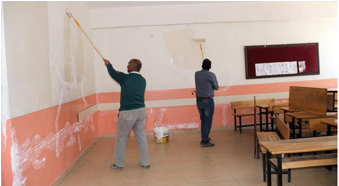
PICTURE 4 Teachers and parents are repairing the public school in city Van, April 2020. (Karaca, 2020)
