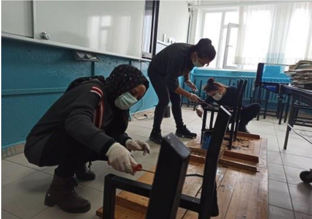
PICTURE 2 teachers were renovating the public school in Samsun in October 2020. (Çokluk, 2020)
