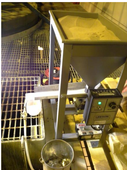
Figure 7. Sand Dosing Feeder
