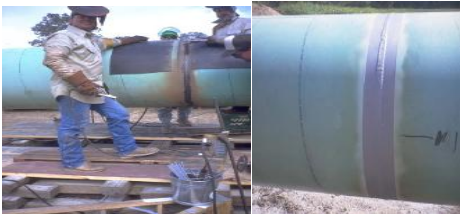
Figure 13. A welding process for two joined steel pipe and already marked steel pipe by welding inspectors' /19/.
