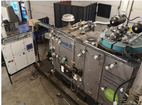
Figure 4. Test boiler in Jamk.
