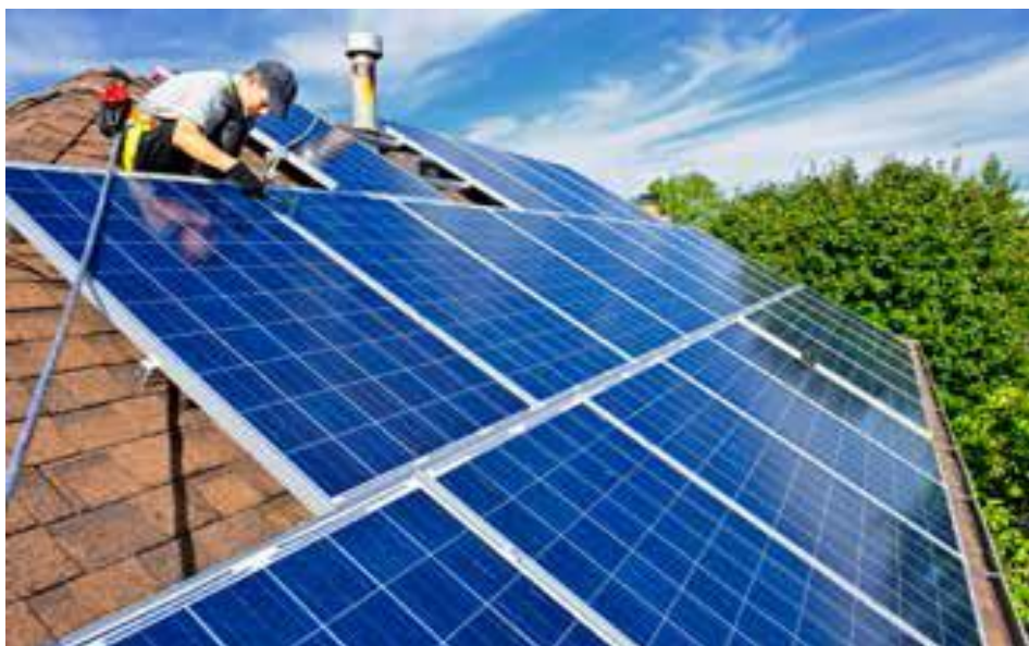
Figure 10: Solar PV panel installed on house roof
