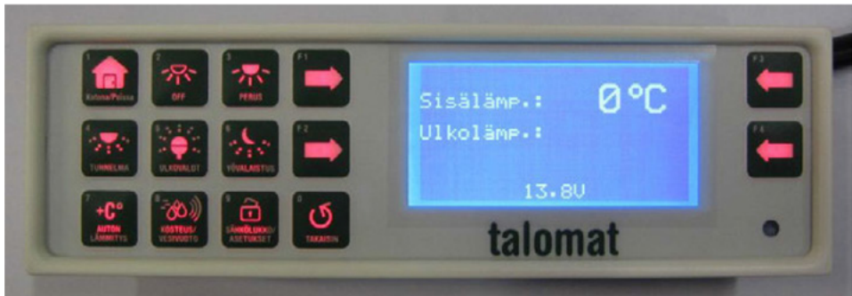
Picture 23. Talomat control panel D92
