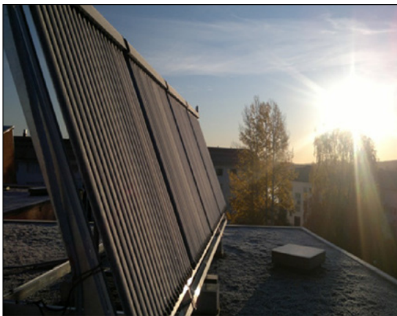
Picture 66. The heat pipes on roof.
