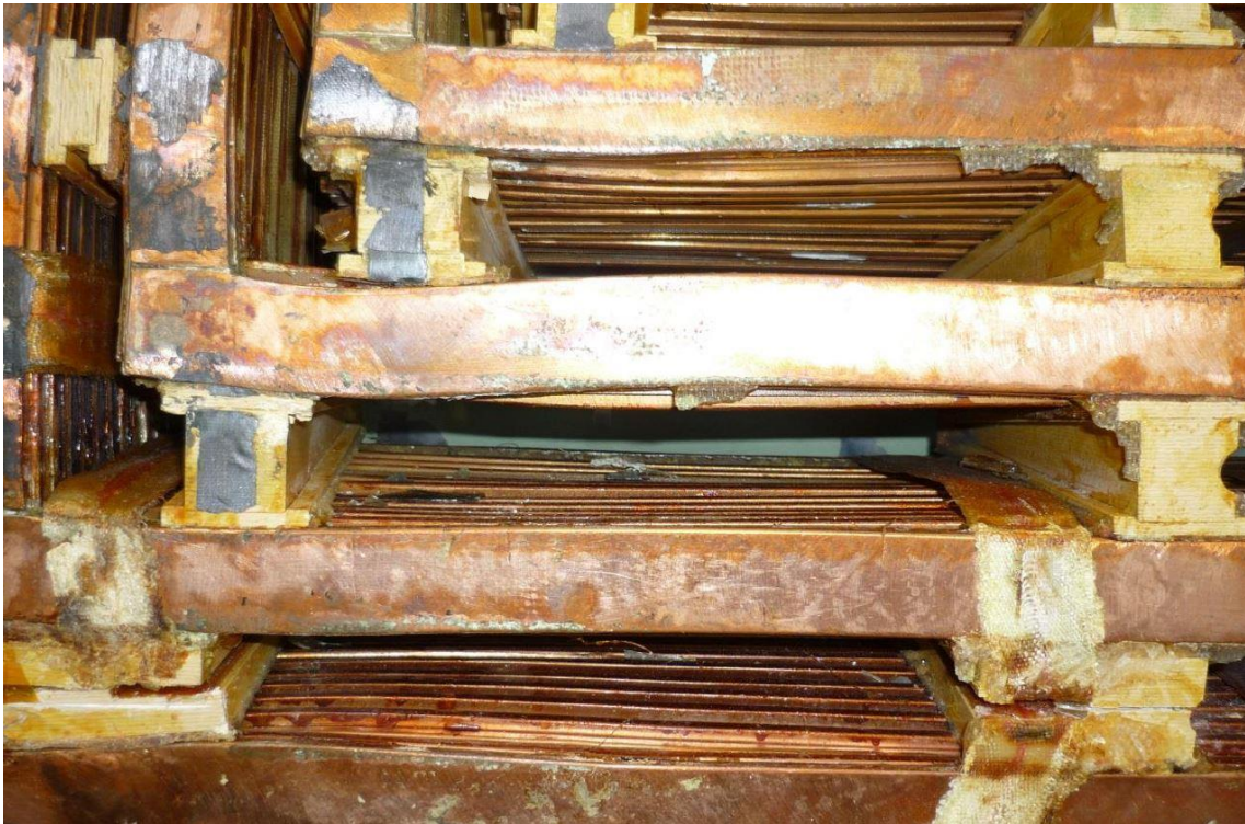
FIGURE 41. Deformed winding head (19)
