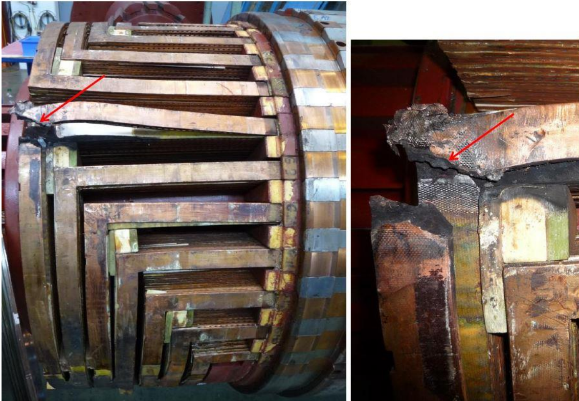
Figure 22. Deformed winding end with cracked soldering joint (19)
