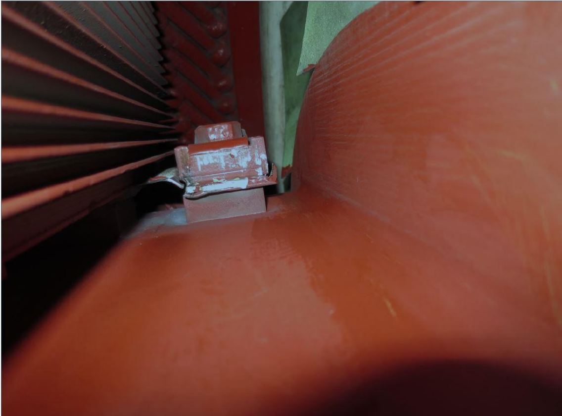
FIGURE 26. A break in the connection point of the rotor pole of salient pole rotor (19)
