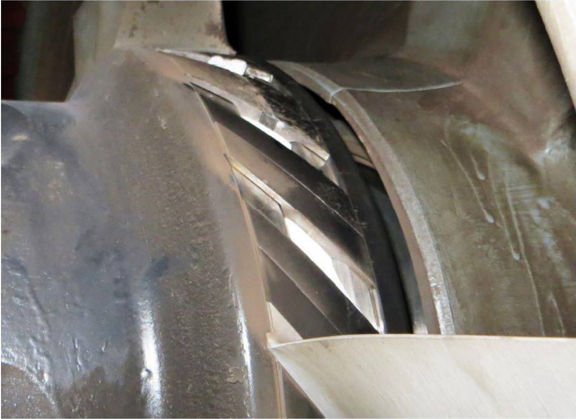
FIGURE 27. Missing blades on the fan (19)
