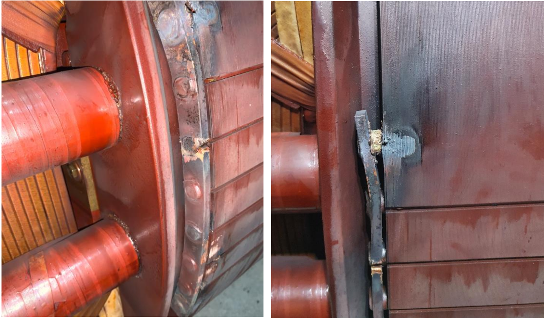
FIGURE 25. Burning marks on the shorting rail, damping rods and pole plate (19)
