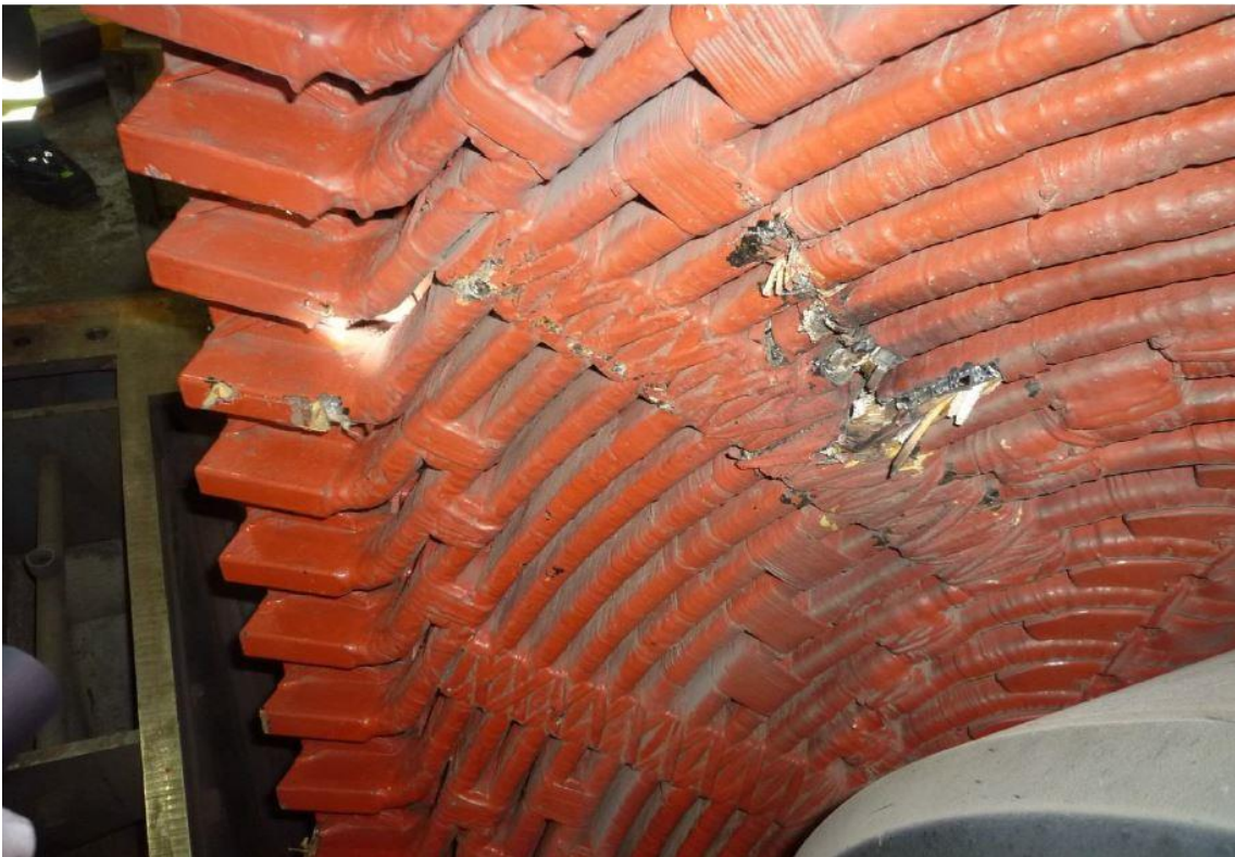
FIGURE 28. Damage in the stator winding caused by the detached fan blades (19)
