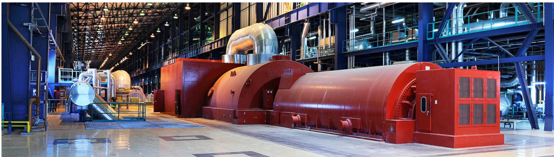
FIGURE 3. Turbo generator header (4)
