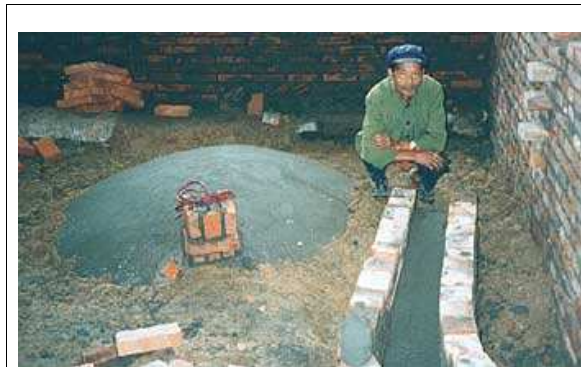
Illustration 2: Completed reactor showing dome top, gas port and toilet and pig pen influent channels at right. Entire structure will be covered with pig pen floor. Picture by Paul Henderson.
