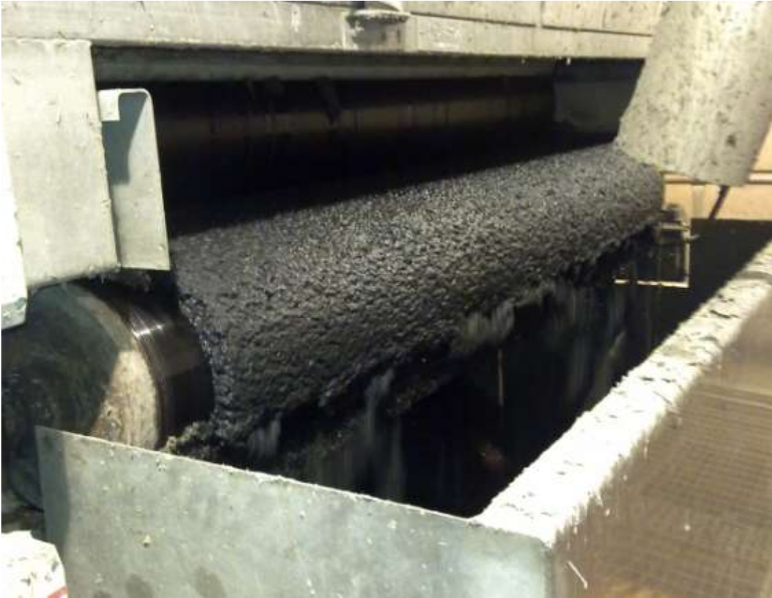
Picture 2. Sludge coming out of the gravity table and dropping to screw dryer.
