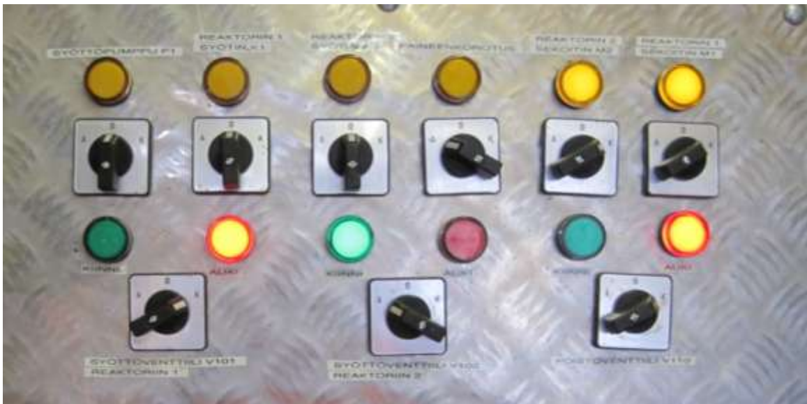
Picture 11. Controlling switches above the touch screen.
