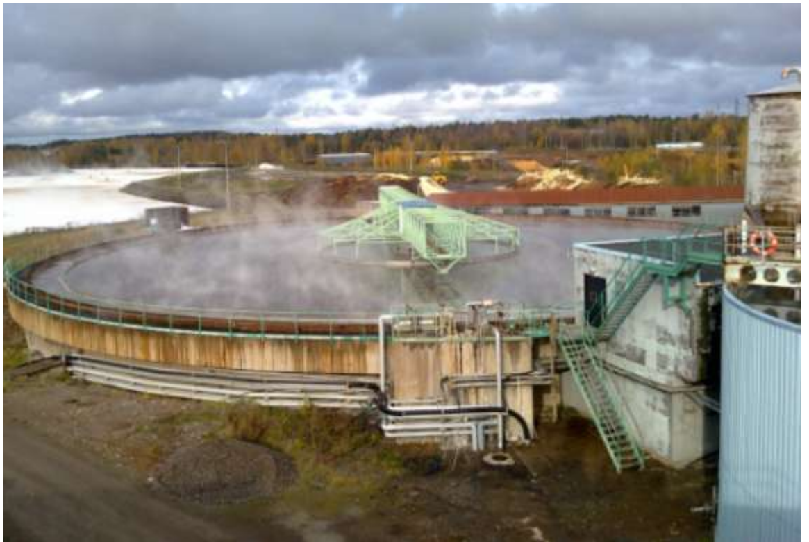
Picture 3. Primary treatment pool with a rotating scraper.
