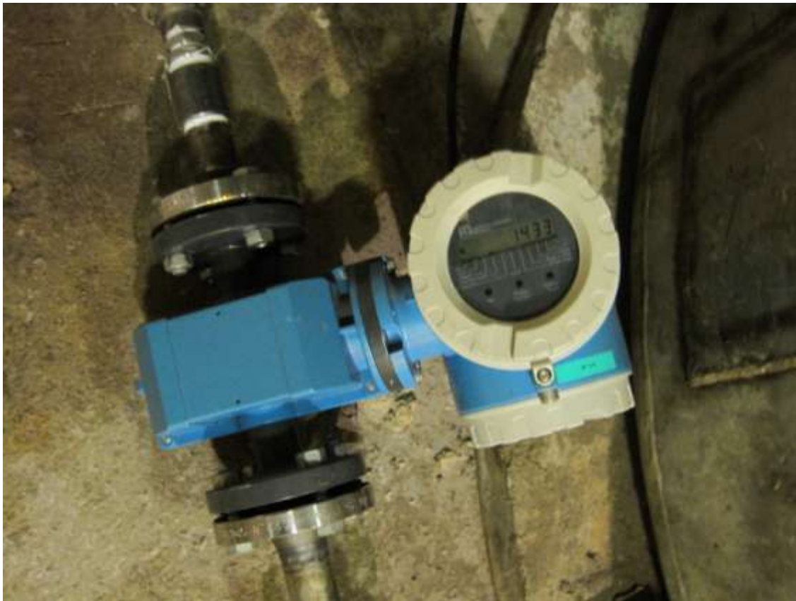
Picture 13. The external flow meter for the sludge to the biogas plant.
