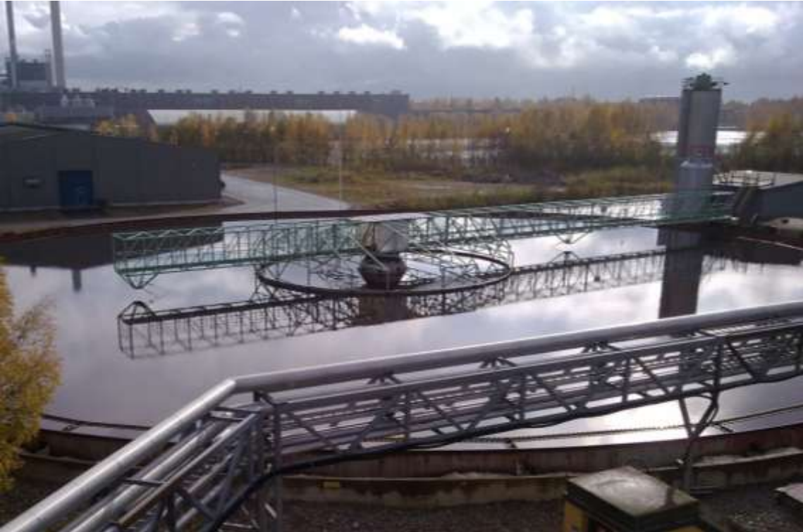
Picture 4. Secondary treatment pool
