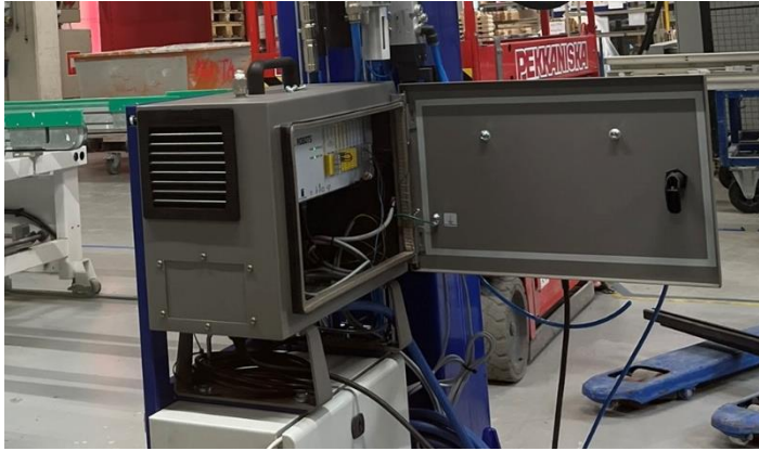
Figure 5.10: Control cabinet showing power supply, and communication cables.
