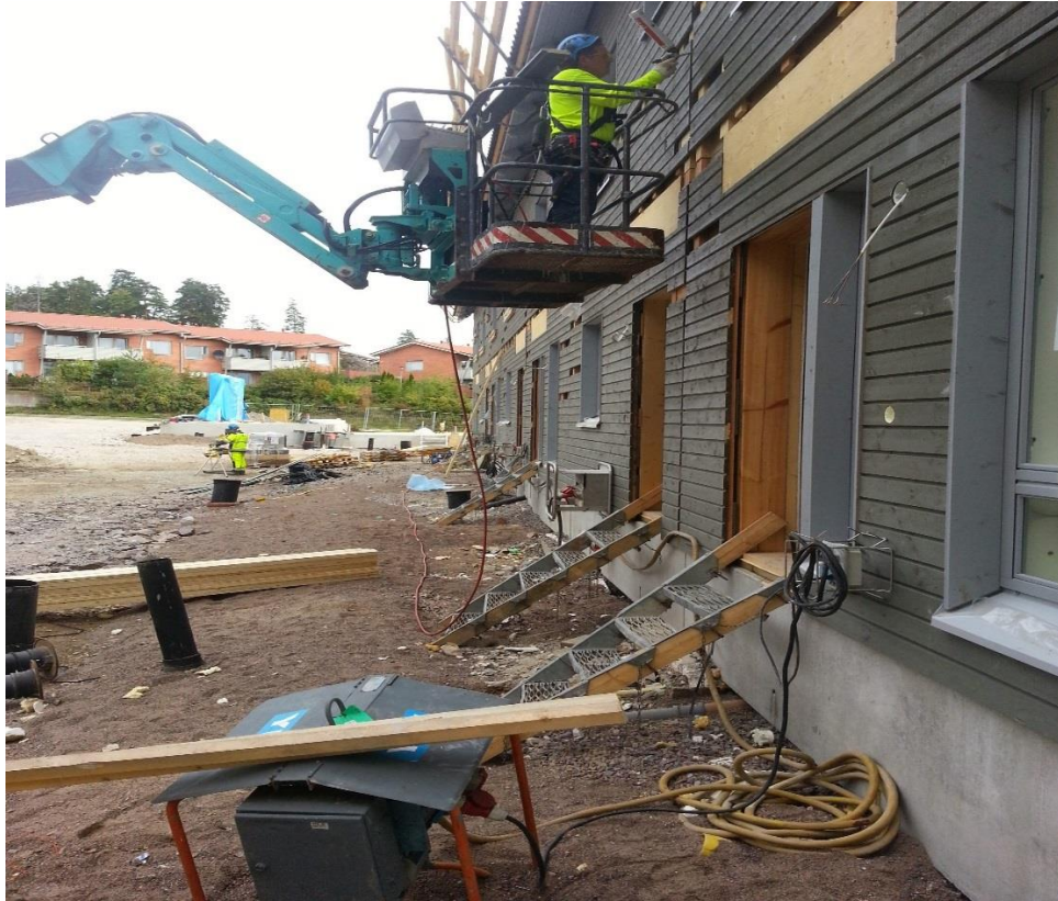
Figure 10 Polyurethane foam sprayed into the vertical seam using a passenger crane. Ahokas M. 2014.
