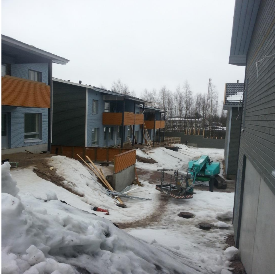
Figure 18 The terrain on the western side of the building B and the eastern ends of buildings D and E. Ahokas M. 2014.
