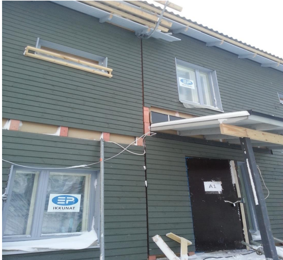
Figure 16 Level difference in A building. Problematic electrical cabling also visible. Ahokas M. 2015.
