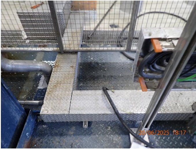
FIGURE 57. Cable tray covered with stainless steel
