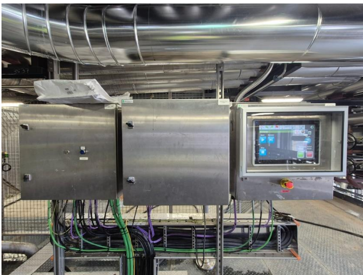
FIGURE 55. Electrical-, pendant- and touchscreen cabinets
