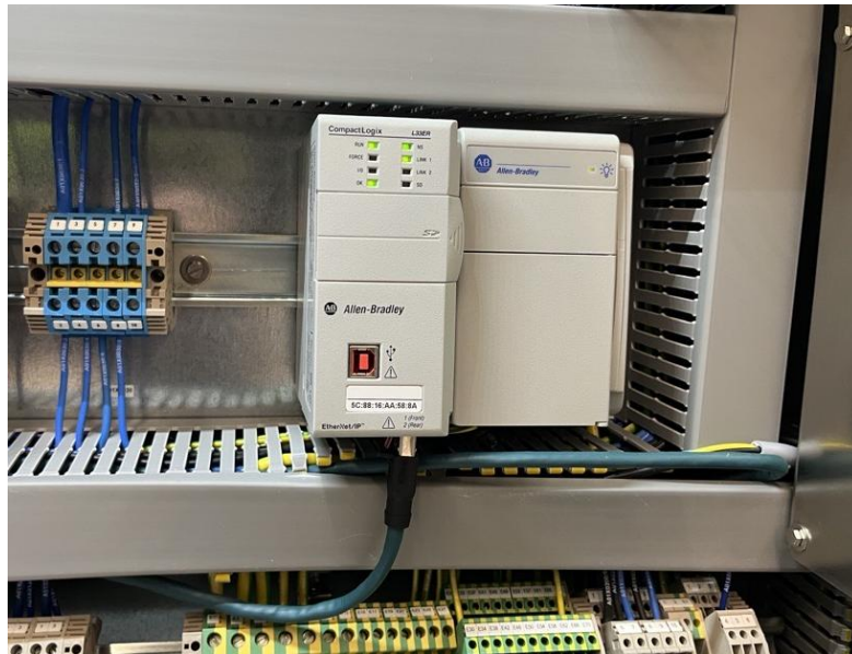
Figure. 15. An Allen Bradley CompactLogix used for testing, which could be the gateway for the proposed IoT energy monitoring system (source: author's own photo).
