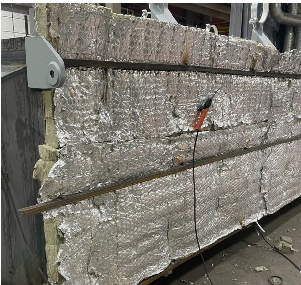
Figure 4. Two vertical support structures are seen welded in place. Photo by author, 2023.
