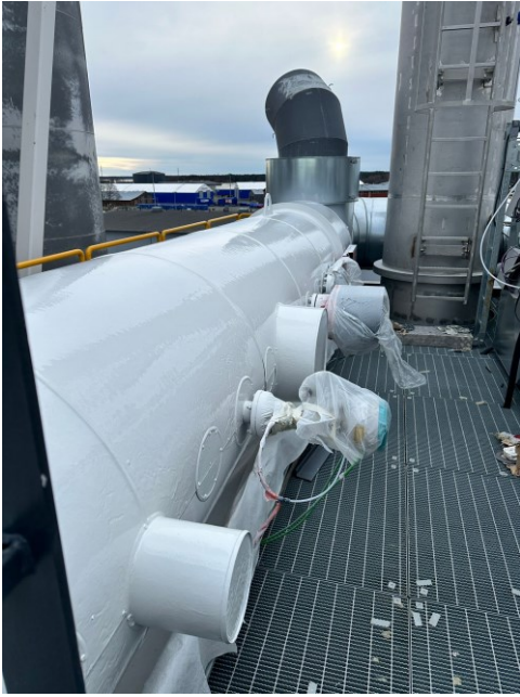
Figure 8. The exhaust gas duct here is seen spray-painted with Geve Therm Safe heat-insulating paint. Photo by author, 2024.
