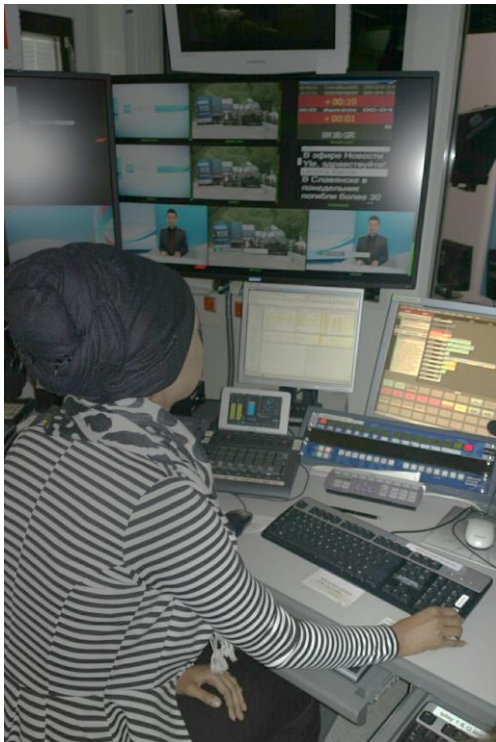
Figure 6. Small control room operation of YLE.
