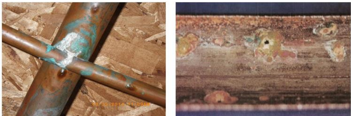
Figure 3. General Corrosion and Pitting Corrosion in a Copper Pipe [16, 17].
