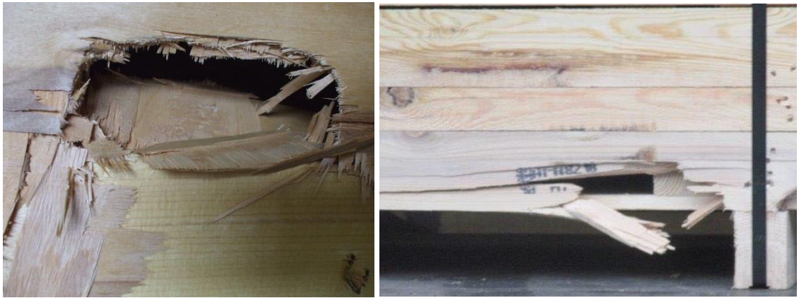
PICTURE 4. Forklift puncture
